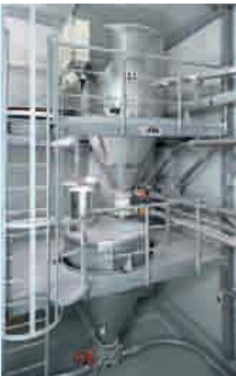
Central weighing station with conveyor scales and buffer container for downstream conveying
