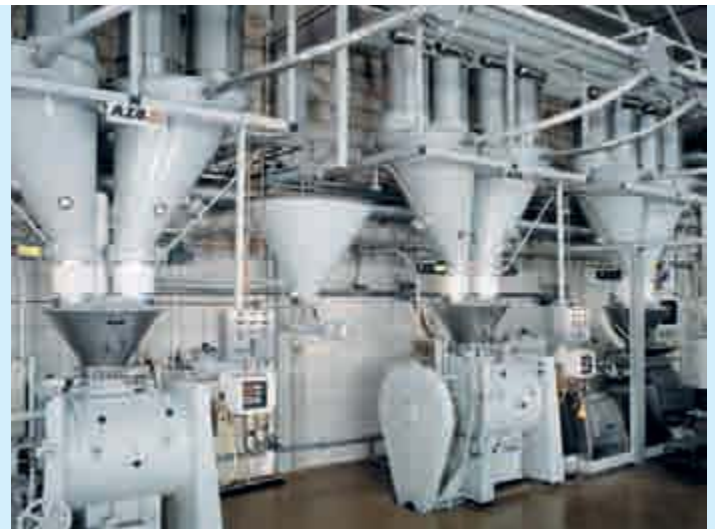
Recipient hopper for flour and sugar in a system with central weighing system
