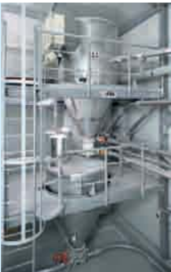
Central weighing station with conveyor scales and buffer container for downstream conveying
