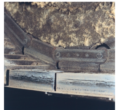
Chain grate furnace
