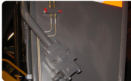
Twin manifold with lube nipple used to fill the bearings on the stick tip and link with lubricant, e.g. after repairs or conversions.
