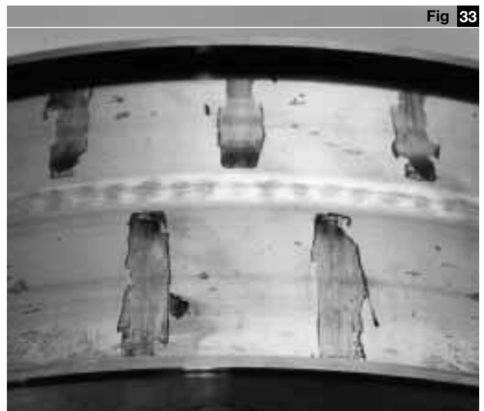
Deep-seated rust under static conditions
